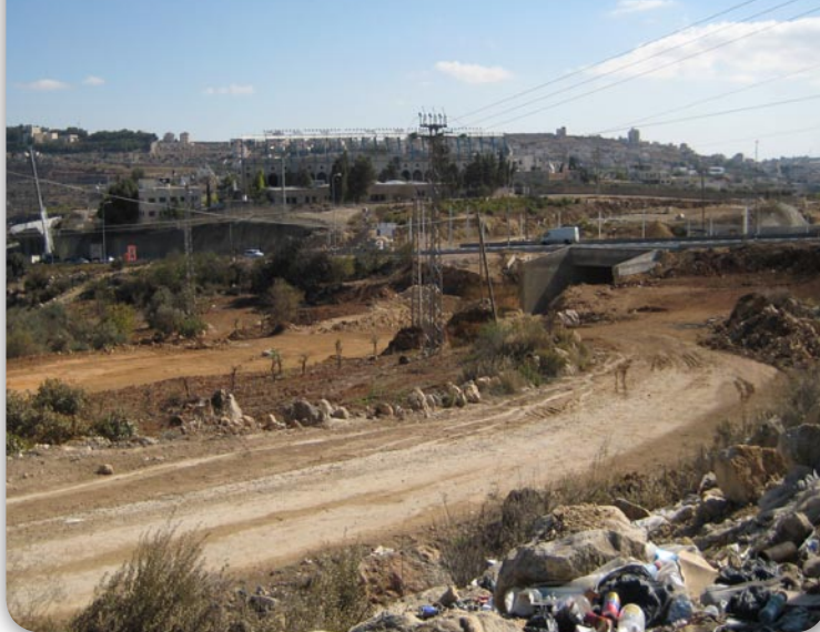
The new road Israel is constructing under Route 60 has run straight through cultivated lands
